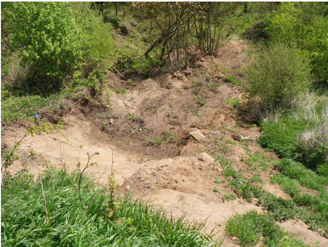
Plate 8 View of mudslide on Knipe Point Headscarp, below Property No. 18 (5 th May 2010) Note continued groundwater issues from slope
