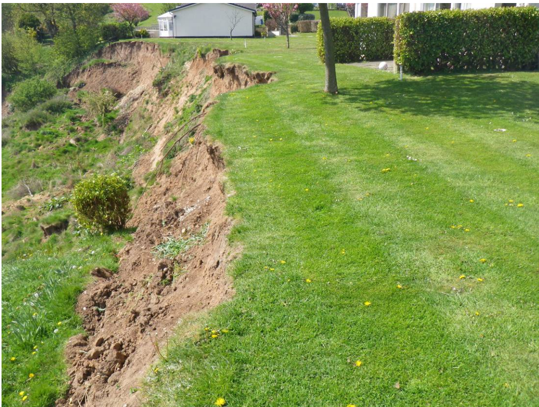
Plate 10 Cliff recession at Knipe Point Headscarp (5 th May 2010)
