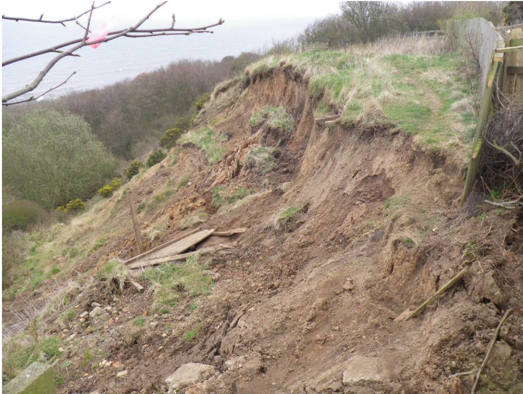
Plate 5 Slope failures on Cornelian Bay side looking east (14 th April 2010)
