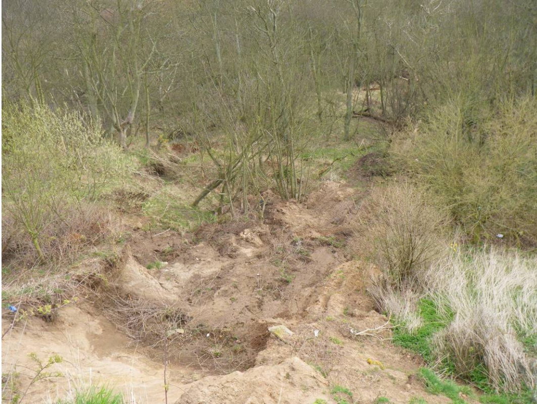
Plate 7 View of 'fresh' mudslide on Knipe Point Headscarp, below Property No. 18 (14 th April 2010) Note groundwater issues from slope
