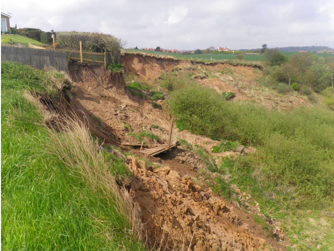
Plate 4 Slope failures on Cornelian Bay side of Knipe Point looking northwest (5 th May 2010)
